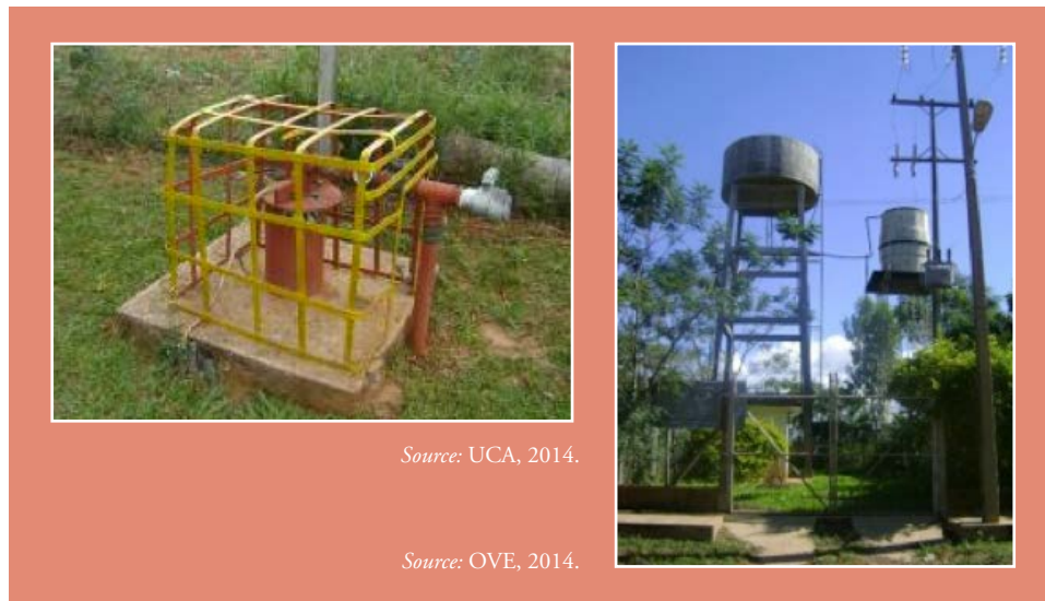
FIGURE 5.1 Well and tank photos
