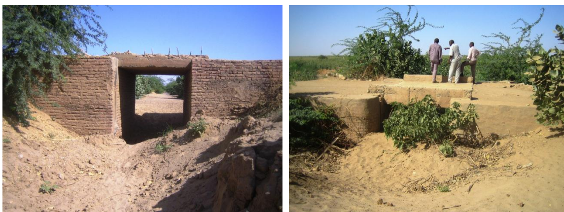
Masga intake structures in Degain block (left) and Kassala block (right) © IFAD/Olaf Verheijen
