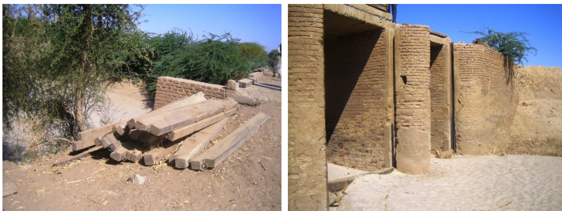
Drop-logs (left) and grooves for installing drop-logs (right) © IFAD/Olaf Verheijen
