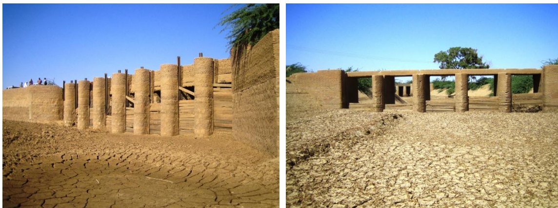
Degain off-take structure with drop-logs (left) and Salam Aleikum off-take (right) © IFAD/Olaf Verheijen
